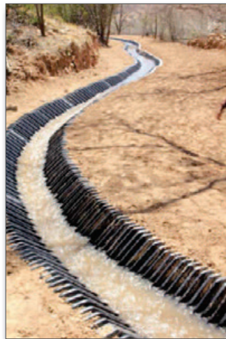
Figure 18. In-ground treatment ditch
