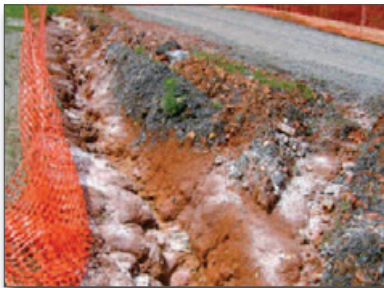
Figure 38. Eroding gully on a construction site
