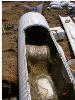
Figure 20. Split pipe with polymer blocks
